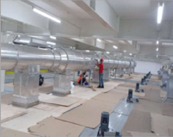
HOT AIR ALUMINIUM DUCTING LINE
